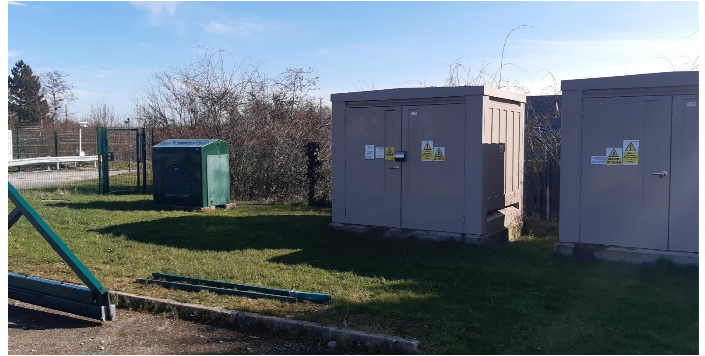
Existing electrical substations adjacent to the vehicle entrance.
