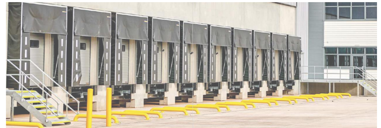
Provision of dock levelling equipment is key to the determination of site levels and floor levels
