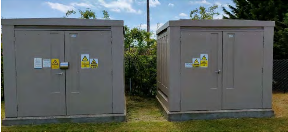
4. Further electrical substation units in the southern tip of the Site.
