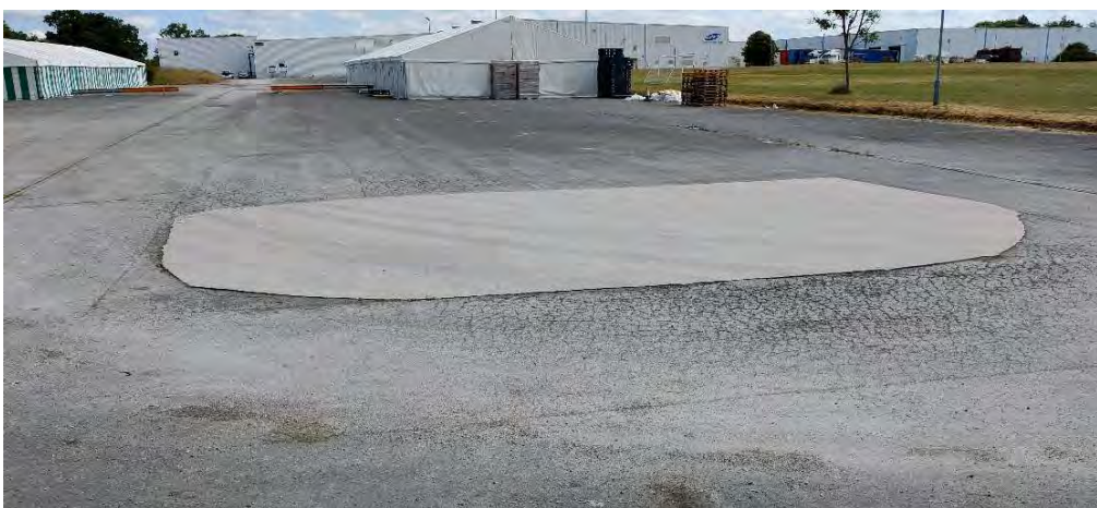
27. Tarmac repair patch on the access road to the north.
