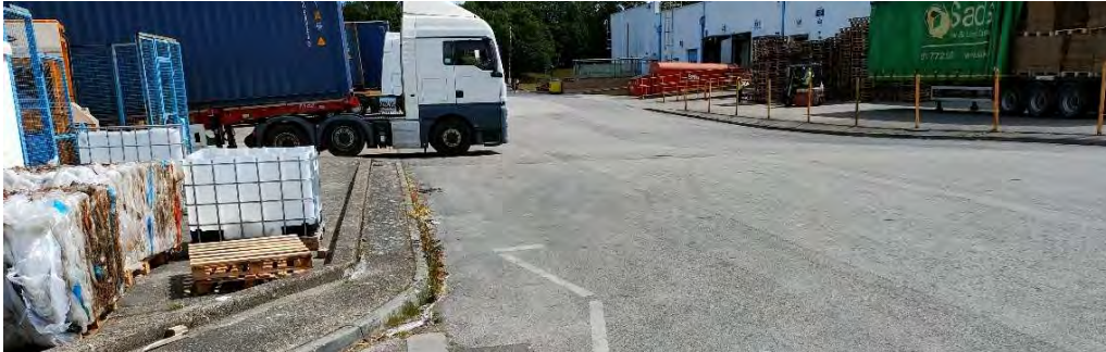
25. Possible subsidence in road noted, which may be underlain by Alluvium deposits. Located away from the proposed warehouse.
